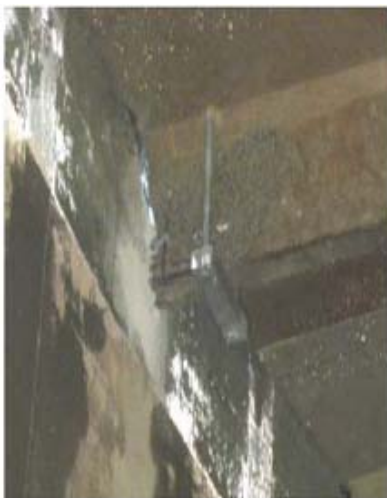
(c)頂板破損
